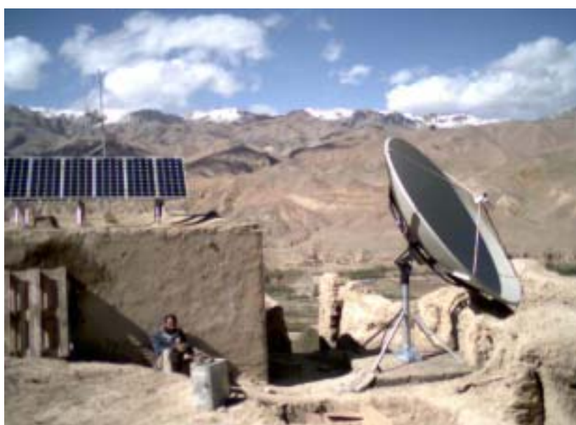
Solar-powered BBC World Service transmitter in Bamian
